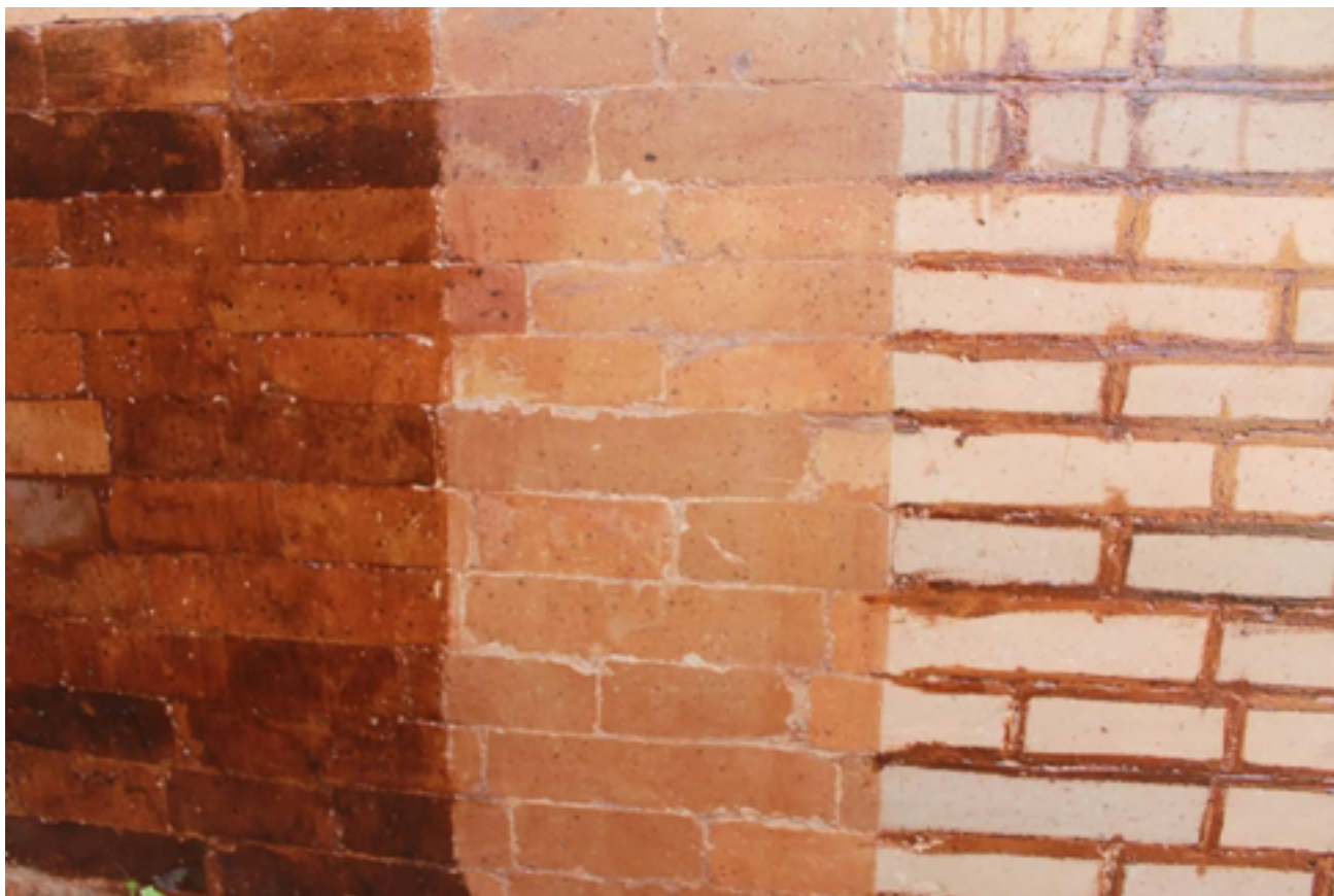
Fig. 6 Direct testing on the body of the Po Rome temple with three different segments. Source: Photo by author, 2012.
